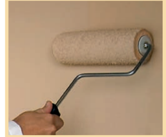
Best results are achieved when the topcoat is applied by an airless spray and then backrolled.
